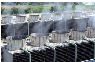
Cooling Tower Energy Saving
