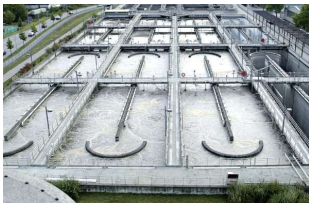
Wastewater, Sewage Treatment
