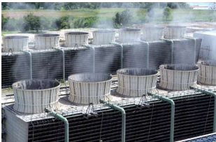
Cooling Tower Energy Saving
