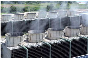
Cooling Tower Energy Saving
